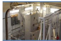
High Pressure Steam 140 kW Boiler 28 kW superheater 5 MPa 427 °C
