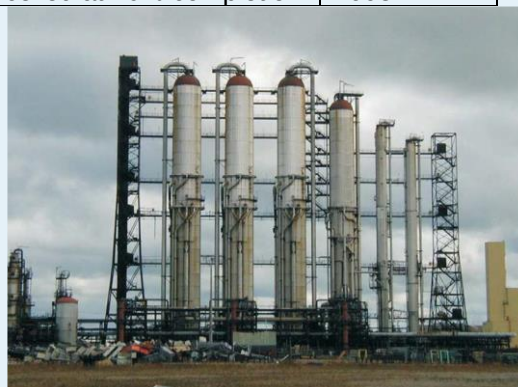
Figure 8: Enrichment unit E4 of plant B (87 m high and 8.5 m in diameter) [31]
